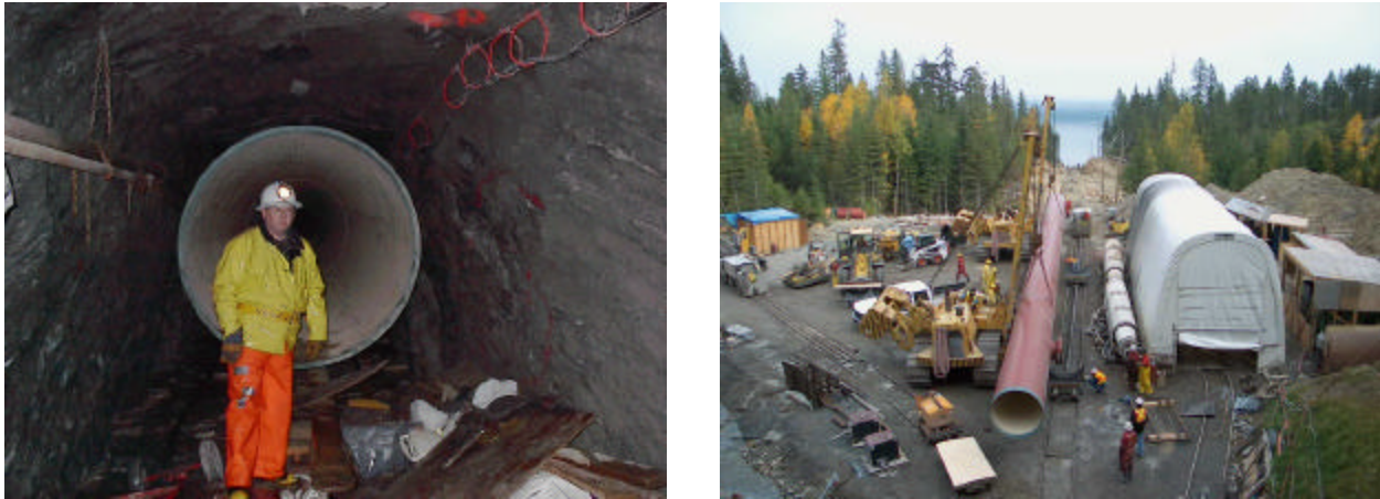
Figure 4: The 1.5 metre diameter penstock in place the lower tunnel (left) and the specialized rail-cart system designed for transporting the 40 m penstock sections into the tunnel with minimal clearance (right).
