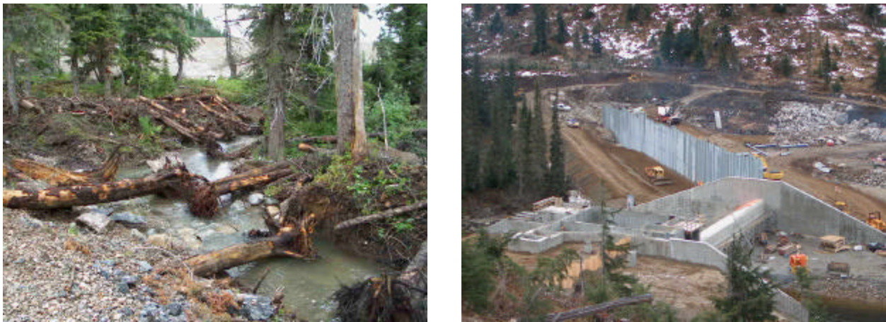
Figure 3: Habitat channels for fish impact compensation (left) and embankment dam under construction upstream (right).
